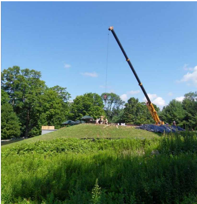
Figure 4. Site protection in place, the crane removing the copings stones from the main roof. (Mary Kay Judy)
