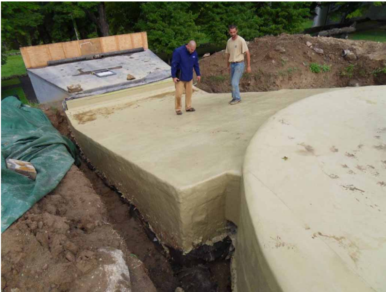
Figure 5. Kemper installed at sub-grade hallway roof and curved edge of main roof. (Mary Kay Judy)
