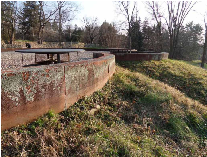
Figure 1. Redstone coping and receding berm at main roof during the investigation phase. (Mary Kay Judy)
