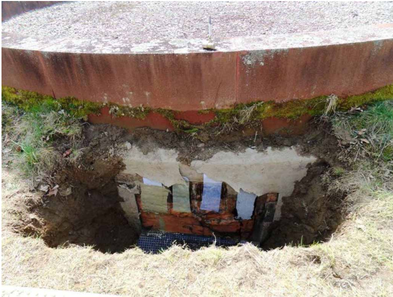
Figure 2. Kemper primer mock-ups at rising wall in trench probe. (Mary Kay Judy)
